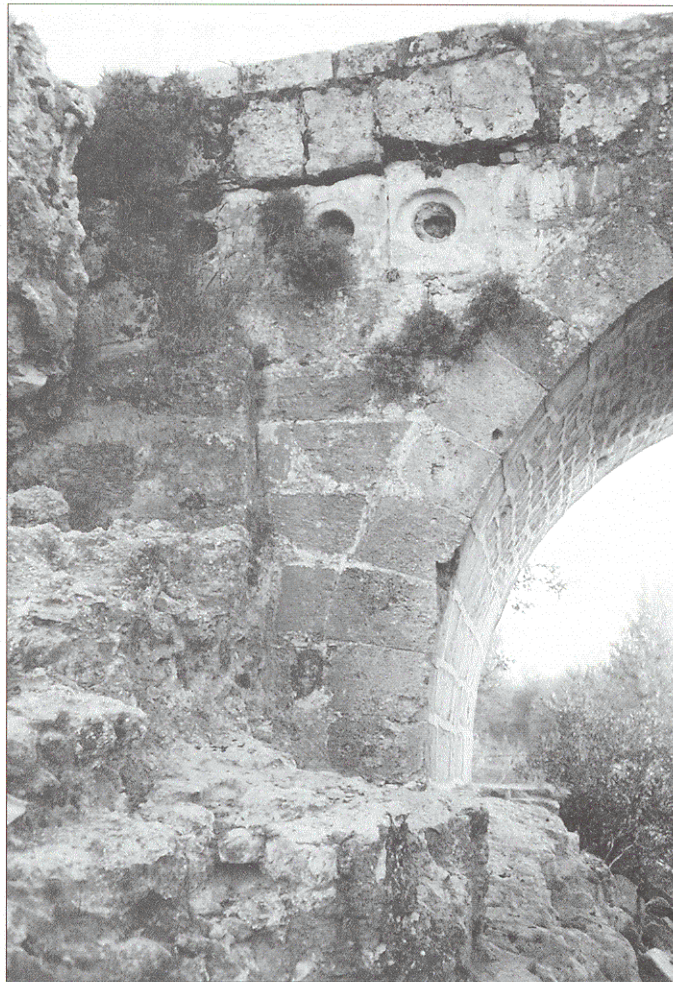
Figure 26 Selçuk bridge over the Eurymedon river, 2 km south of Aspendos, incorporating stone pipe elements of the siphon.
